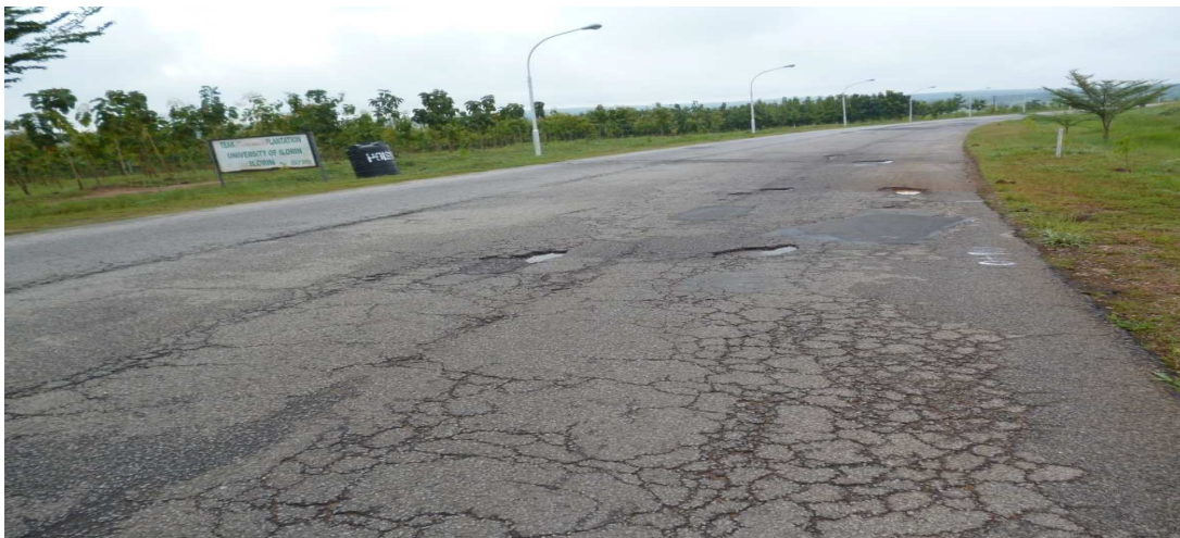
Figure 2.3: Cracking, potholes and raveling
