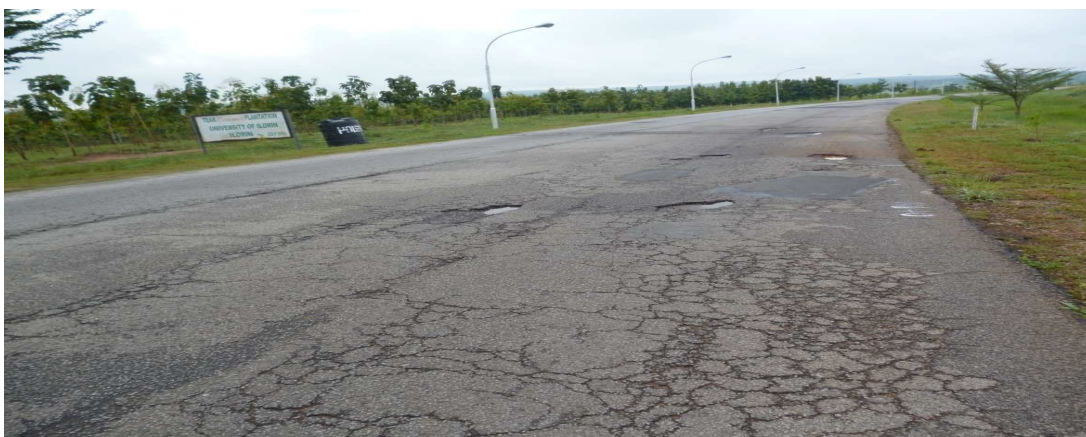
Figure 2.2: Cracking and potholes
